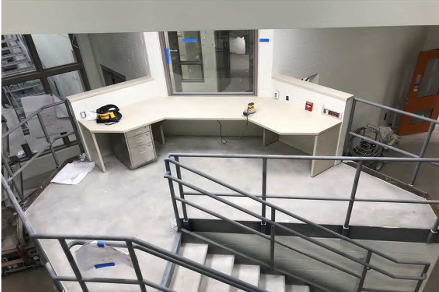
2 nd Floor Local Control Platform
