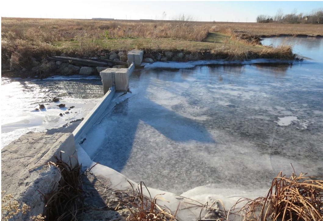
Ice forms behind the new steel gates in the Phase 1 marsh. Water levels will be three to five inches deeper in this marsh during 2015 (average depth will be 10 to 13 inches).
